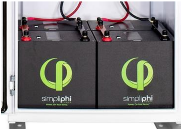
Figure 9.0 – Interconnecting Busbars Parallel the Batteries in Sets of Two
