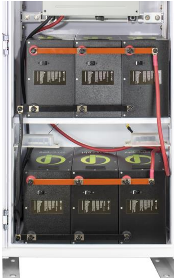
Figure 11.0 – Six-PHI Battery Orientation within the Sol-Ark-12K-22.8 kWh
